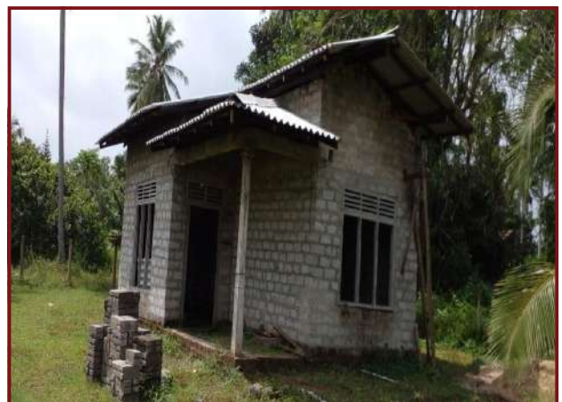
A house being constructed at Horathapalawa for disabled migrant worker, Mrs. A. A. D. Wijayanthi
